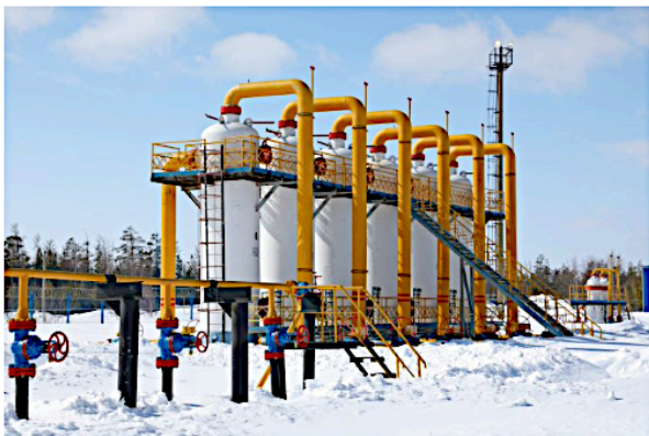
Natural gas storage facility in Russia
